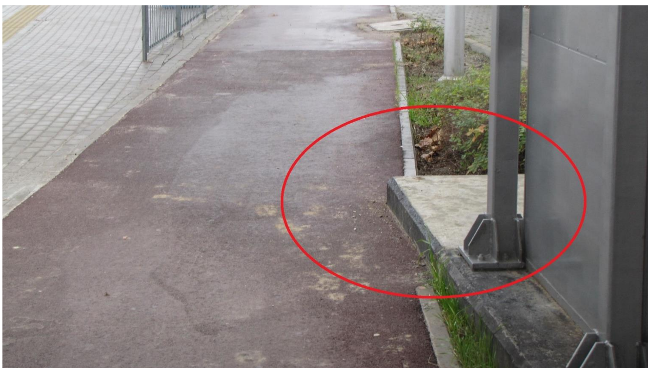
Figure 5. The eastern section of the S8 expressway in Warsaw, Poland was equipped with cycling facilities, but because of lack of enforcement of quality requirements the cycle tracks are not safe to use.
