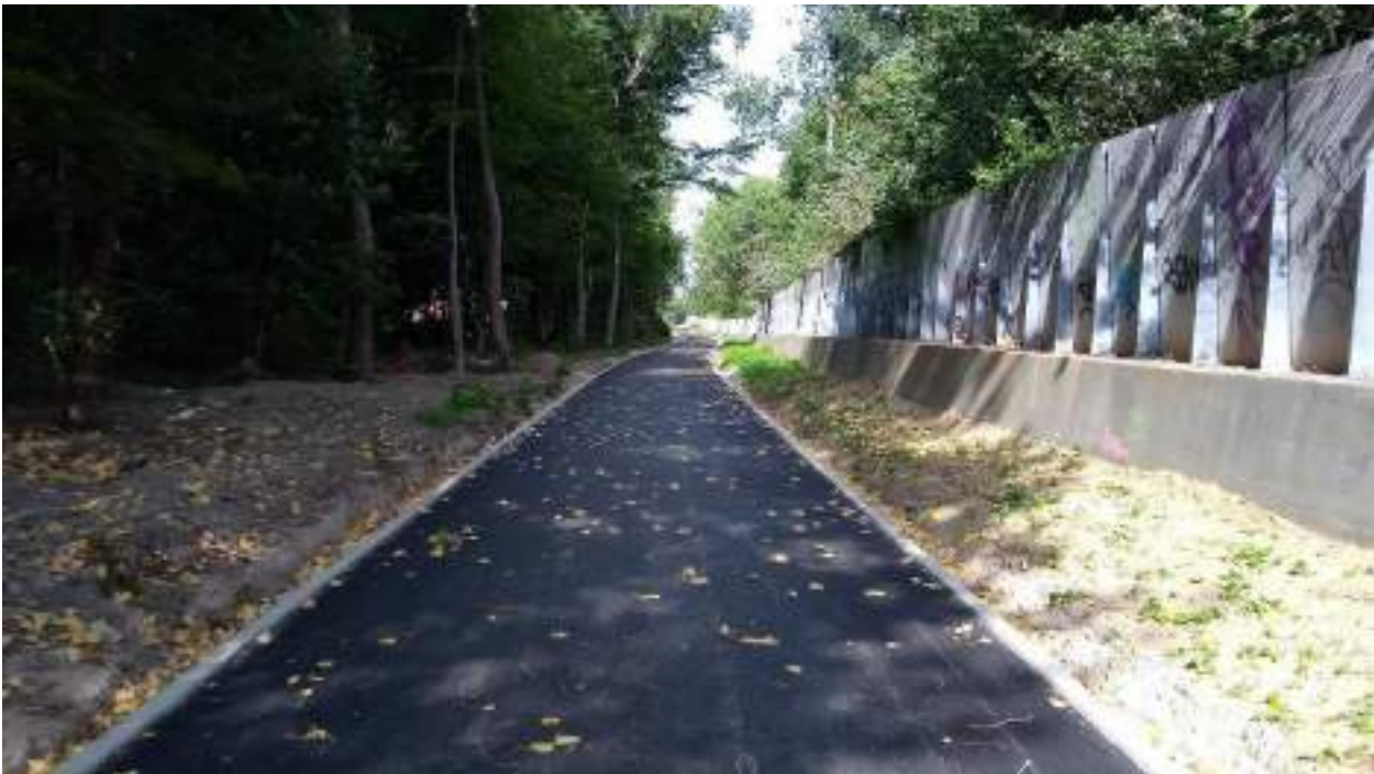
Figure 43. Construction of the F203 cycle highway along the E40 motorway to the east of Brussels. The motorway is behind the noise barriers on the right.
